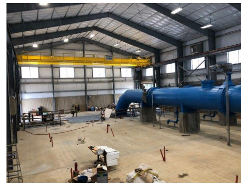
Kennedale Balancing Reservoir Pressure Control Station
