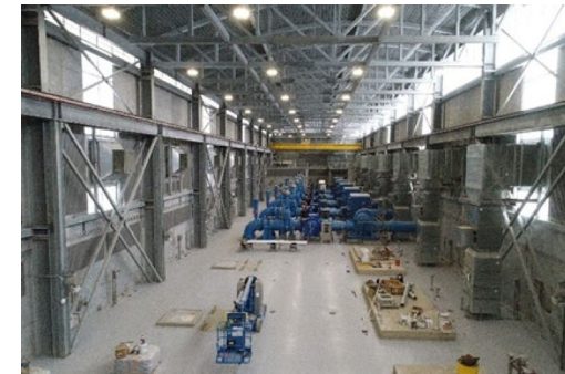
Joint Booster Pump Station 3 (JB3)
