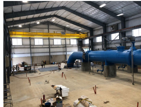
Kennedale Balancing Reservoir Pressure Control Station
