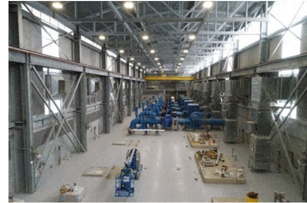
Joint Booster Pump Station 3 (JB3)
