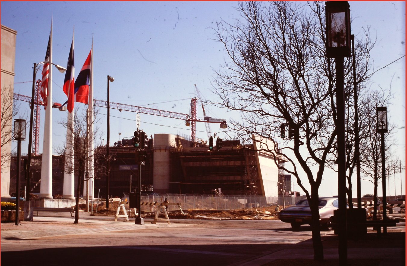
City Hall under construction, 1974. Image courtesy of the City of Dallas historic preservation team.
